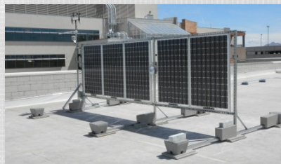
Testing bifacial PV panel to search for an accurate electrical circuit model.
