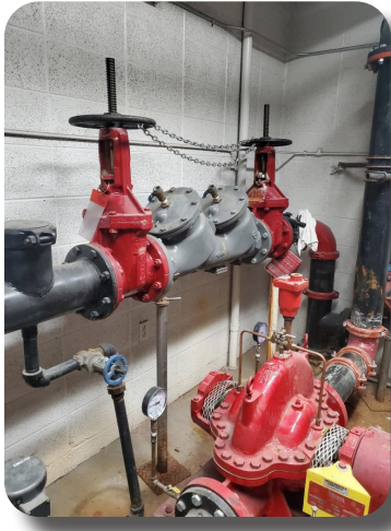
Picture Above: Before at BEH-Fire Pump room
